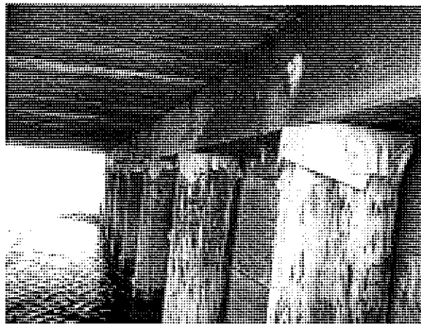
Sample L-2. Lead sample from Abutment pile cap at SE corner of bridge. Typical all abutment and pier piles.
