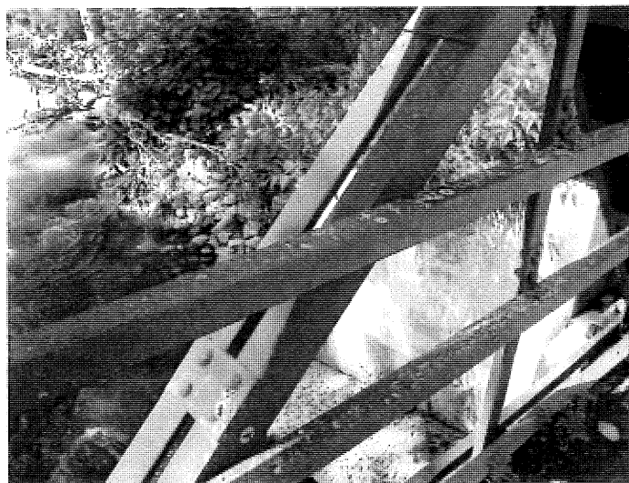
Sample LP-2. Lead paint sample from bridge rail on upstream side, North end of bridge.
