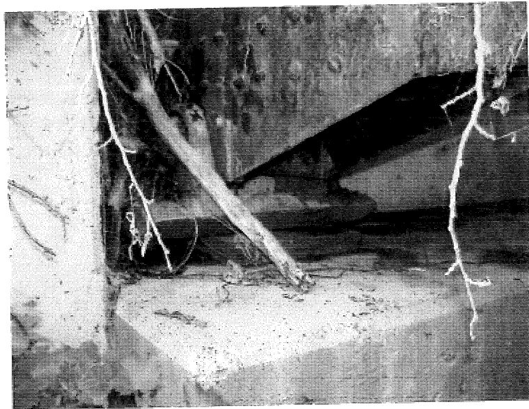
Sample LP-1. Lead paint sample from abutment girder near rocker pin assembly. SW corner of bridge.
