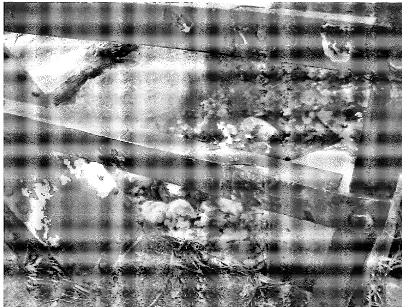
Sample LP-3. Lead paint sample from railing at SW corner of bridge.
