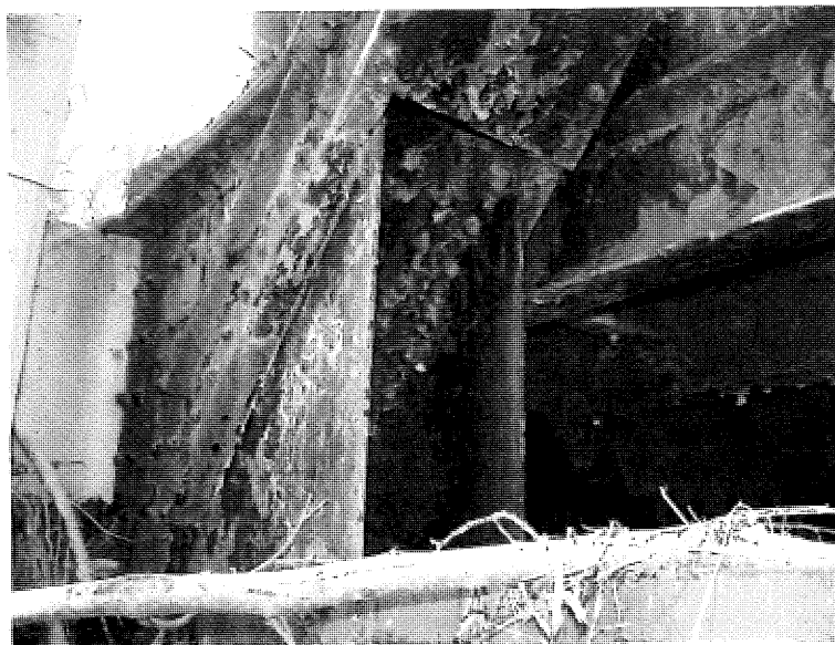
Sample LP-6. Lead paint sample from truss member at NE corner of bridge.
