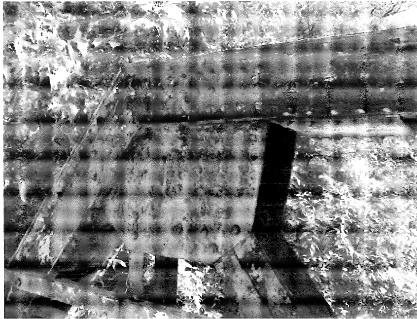
Sample LP-5. Lead paint sample from gusset plate at NE corner of bridge.
