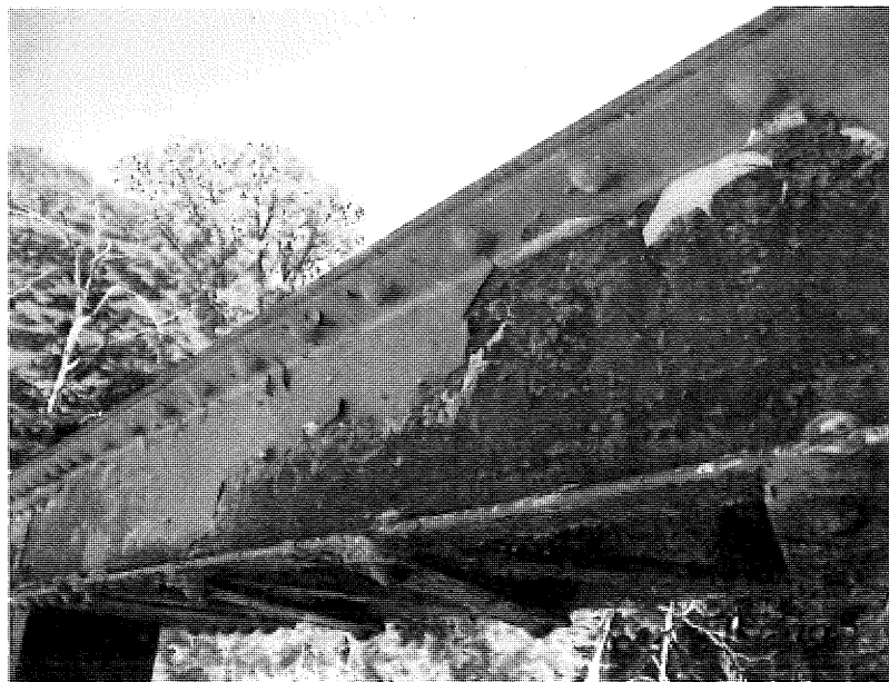
Sample LP-6. Lead paint sample from top truss member, South side at midspan.
