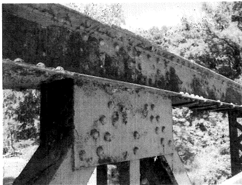
Sample LP-3. Lead paint sample from truss member. Downstream side of bridge at midspan.
